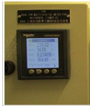
Photo 1: A metering device for a 400A circuit
