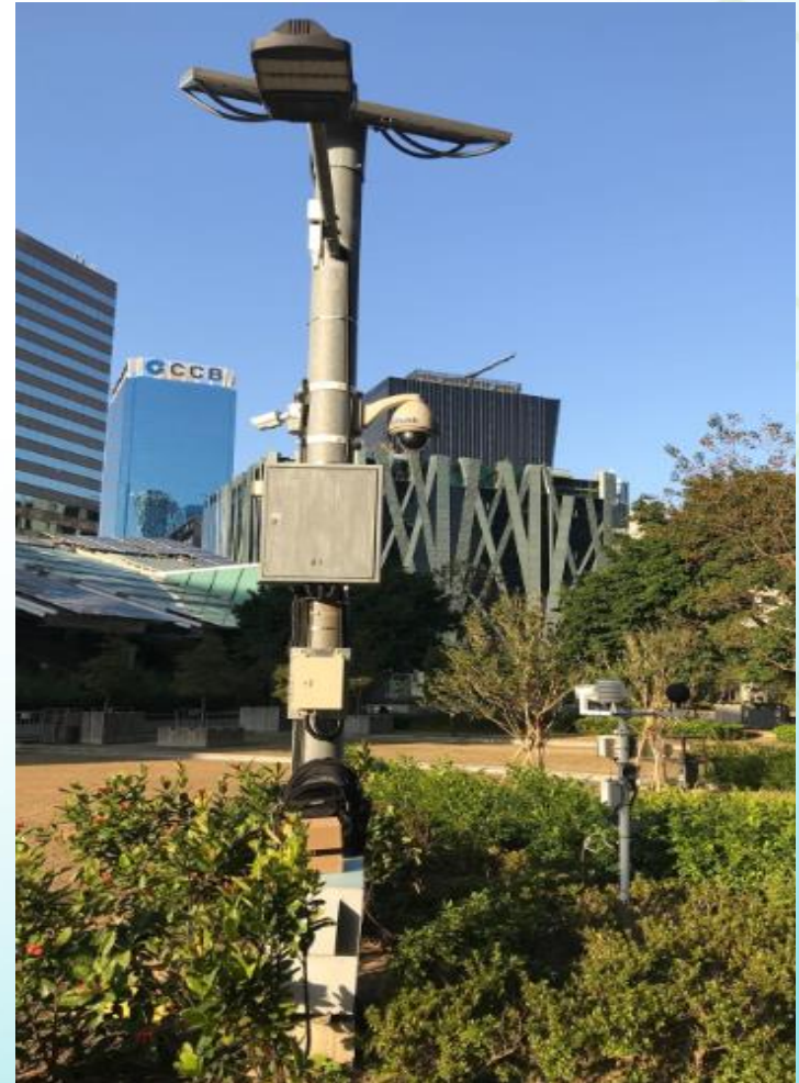
Location A - A set of sensors for measuring wind, temperature and humidity
